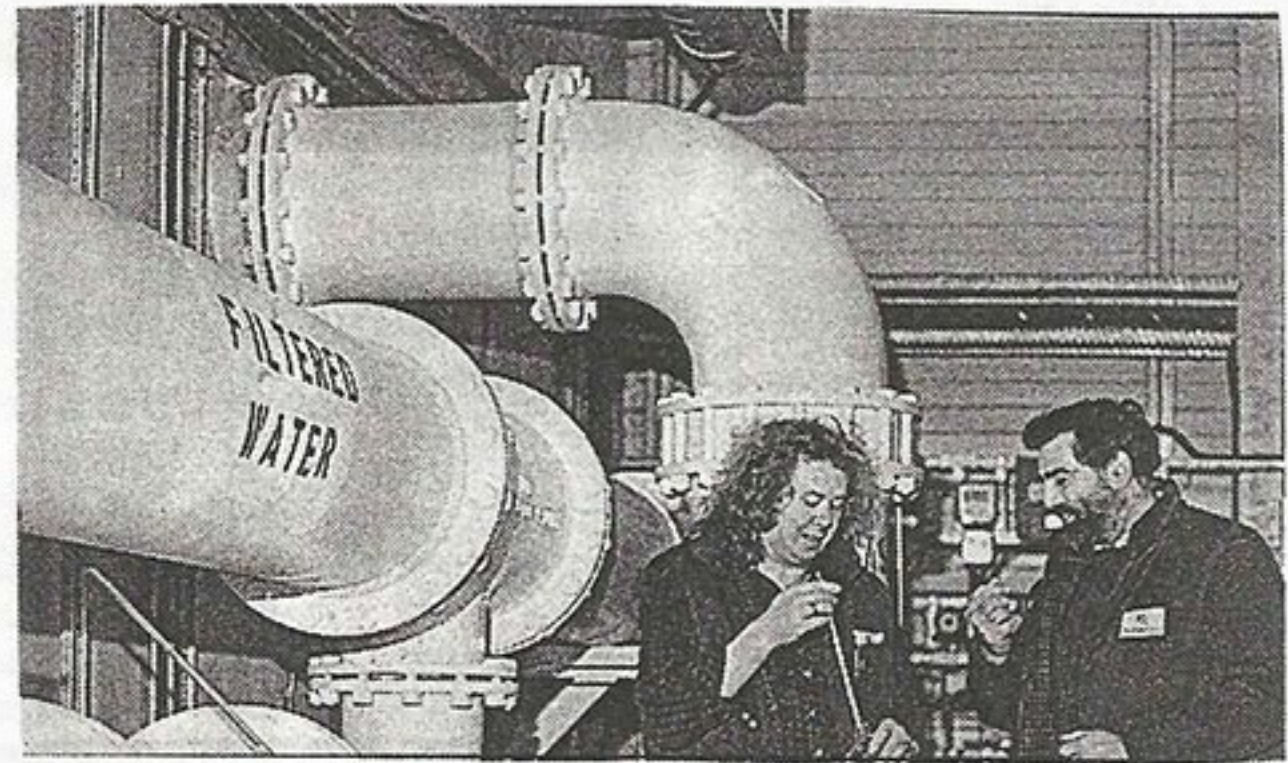
Inside, the plant is a maze of pipes and hoppers
